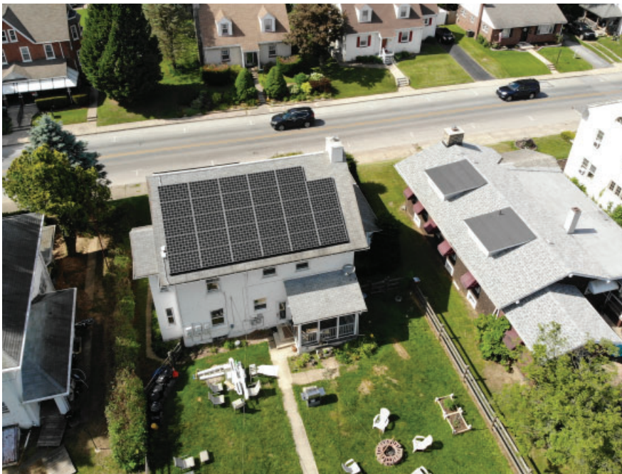
An example of a home in Parkesburg Borough where solar panels were installed to increase energy efficiency
