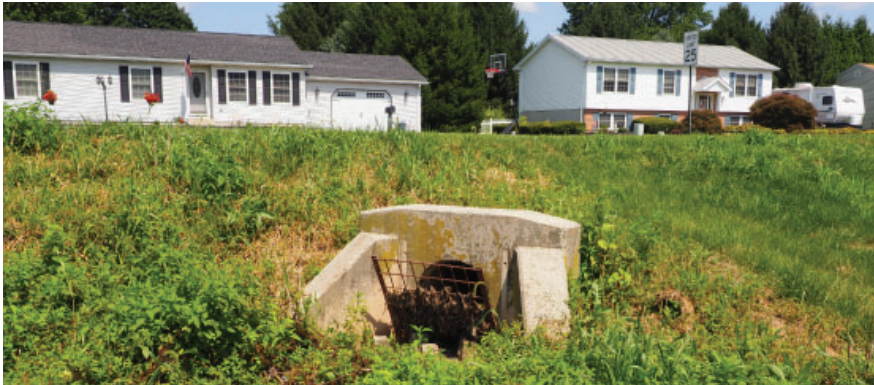
Aging stormwater management facility in the southwestern corner of the Borough
