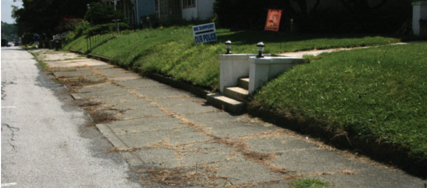
Sidewalk in need of repair or replacement on 1st Avenue near East Bridge Street
