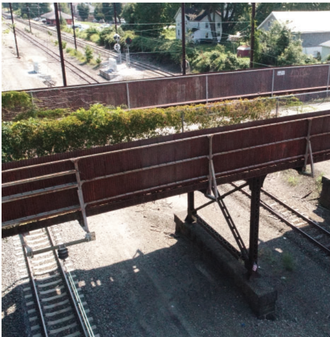
The West Bridge Street Bridge will provide a vital vehicular and pedestrian link between the Northside and Southside of the Borough
