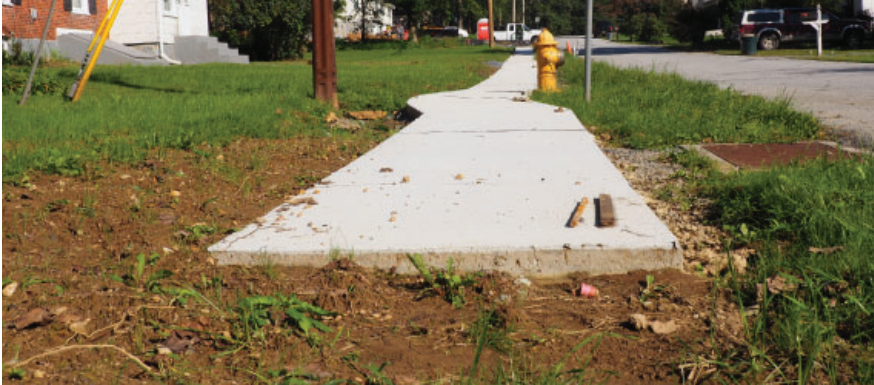
An example of a missing link in the Borough's pedestrian network
